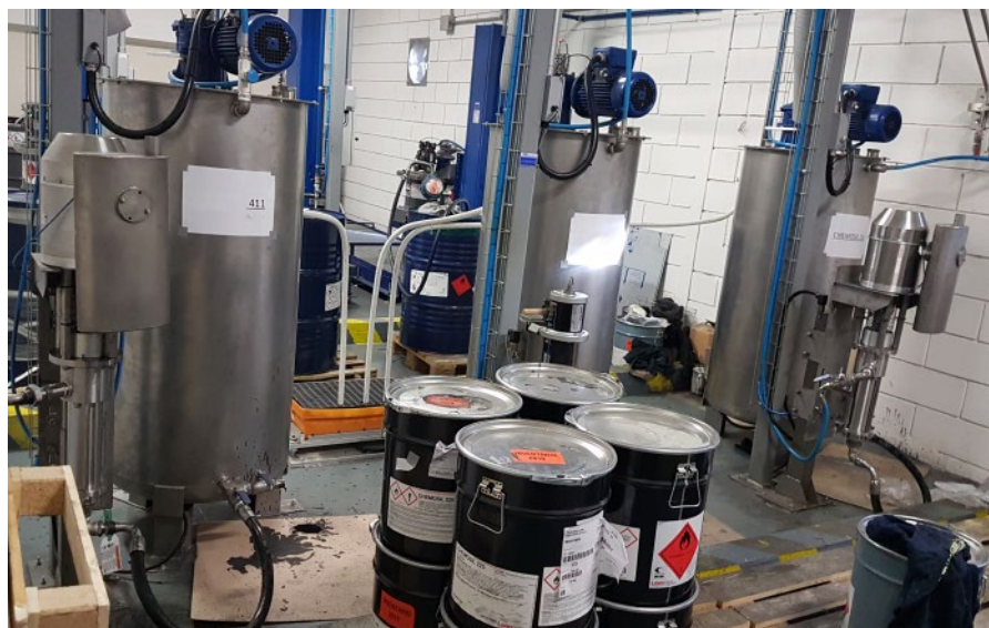
Complete mixing equipment Centralized pumps supply system for feeding to automatic coating machine (rigid line expansion up to 900 mt)
