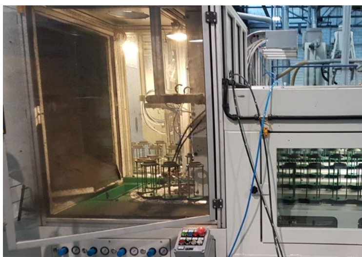
Coating machine direct connected to centralized plant.
