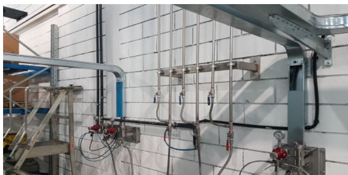
Delivery and recirculation line close to coating machine.
